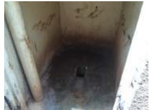
A toilet stall—nothing but a hole in the concrete floor
