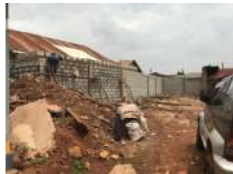
The water channel is on the other side of this new wall
